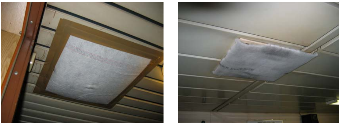
Figure 10: Supply air terminal unit with dishcloth (left), and with filter material (right).
