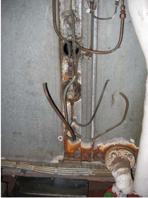
Figure 11: Hygiene deficiencies on a humidifier.
