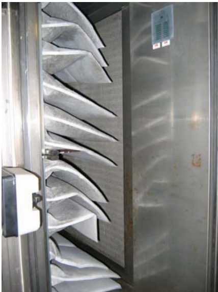
Figure 12: Installation of a bag filter with face contact with the floor of the chamber
