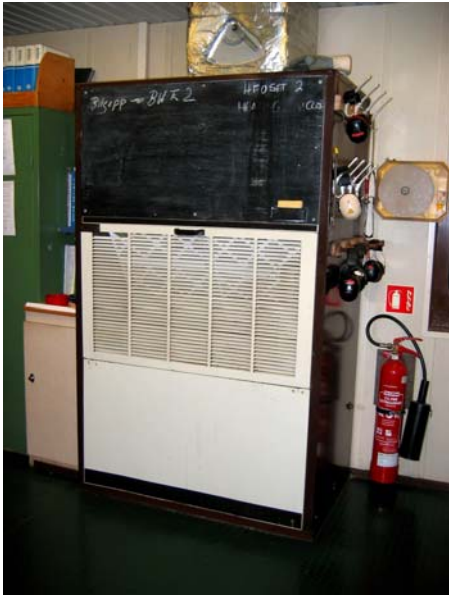
Figure 2: Air-refrigeration system in an engine control room.
