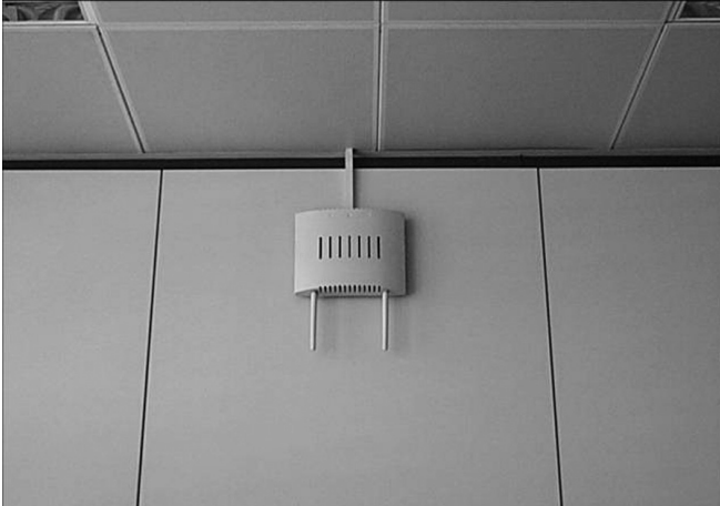
Figure 18: Access point for DECT systems
